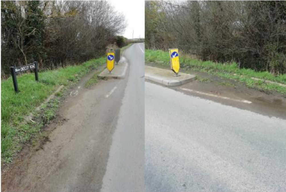
Poorly Maintained and Dangerous Cycle Bypass
